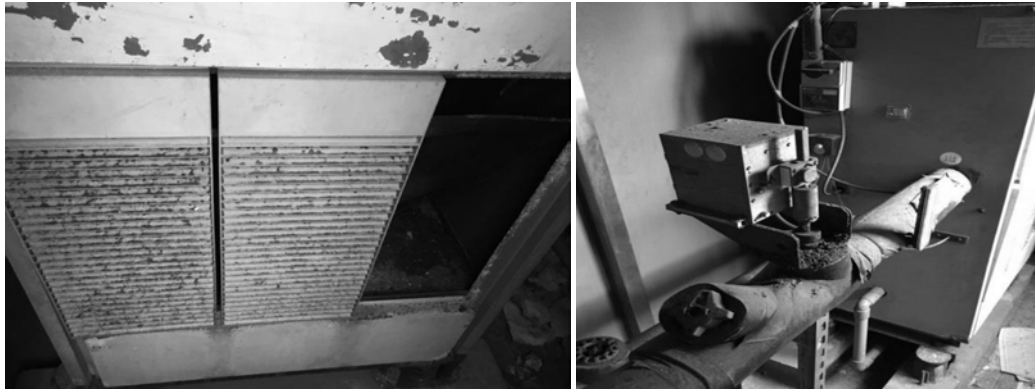
Figure 4. Conditions of make-up air unit (MAU)
