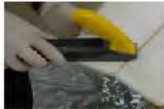
(e) Laminating resin stays tacky and is unsandable so sur-form is used to smoothen the rough surfaces
