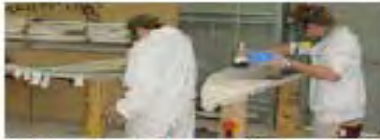
(l) Catalysed filler resin & sanding resin was applying on deck, left, and bottom part, right, of the surfboards
